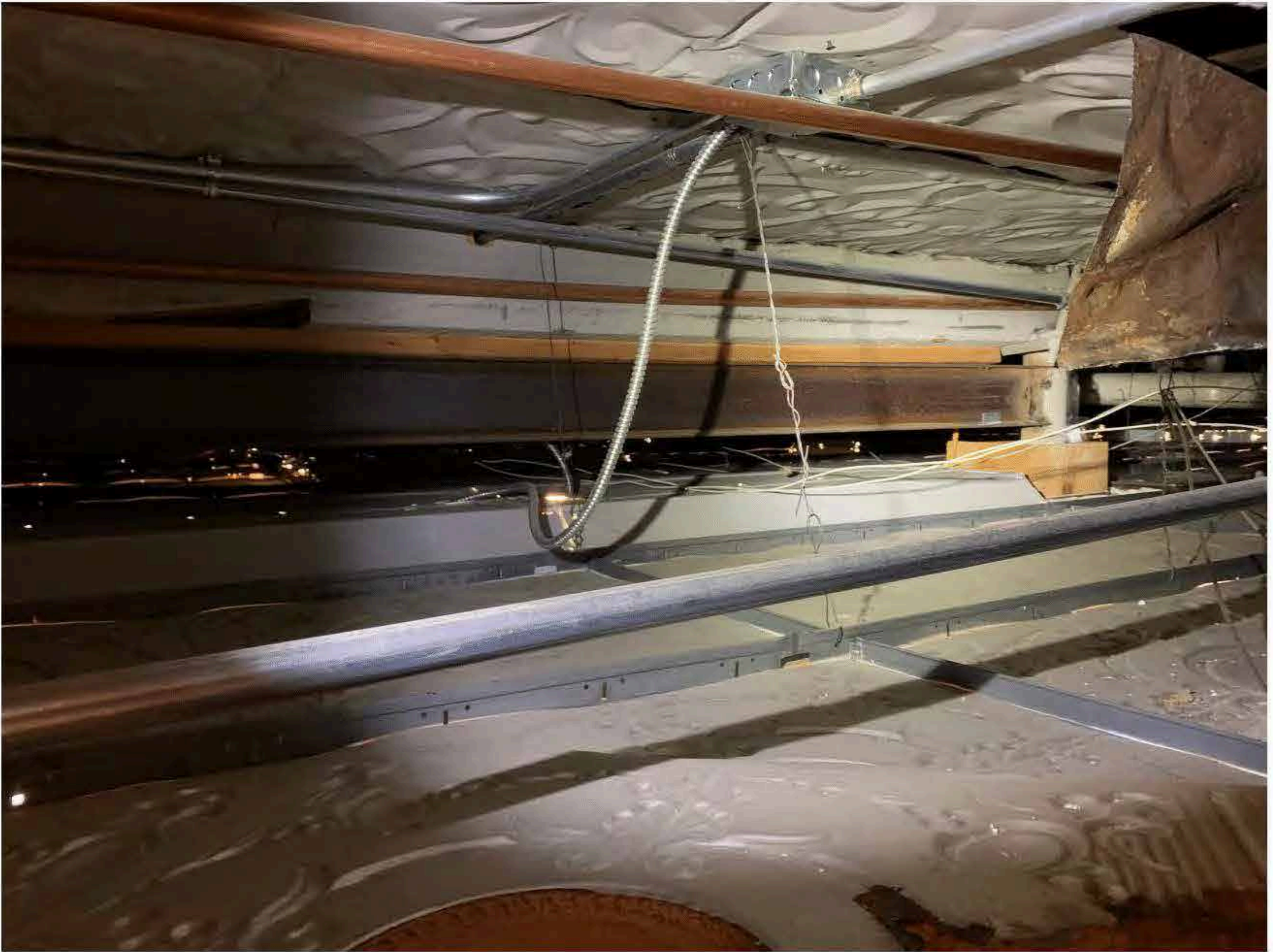
Figure 3.8-3: Main level conduit runs and lighting at dropped ceiling
