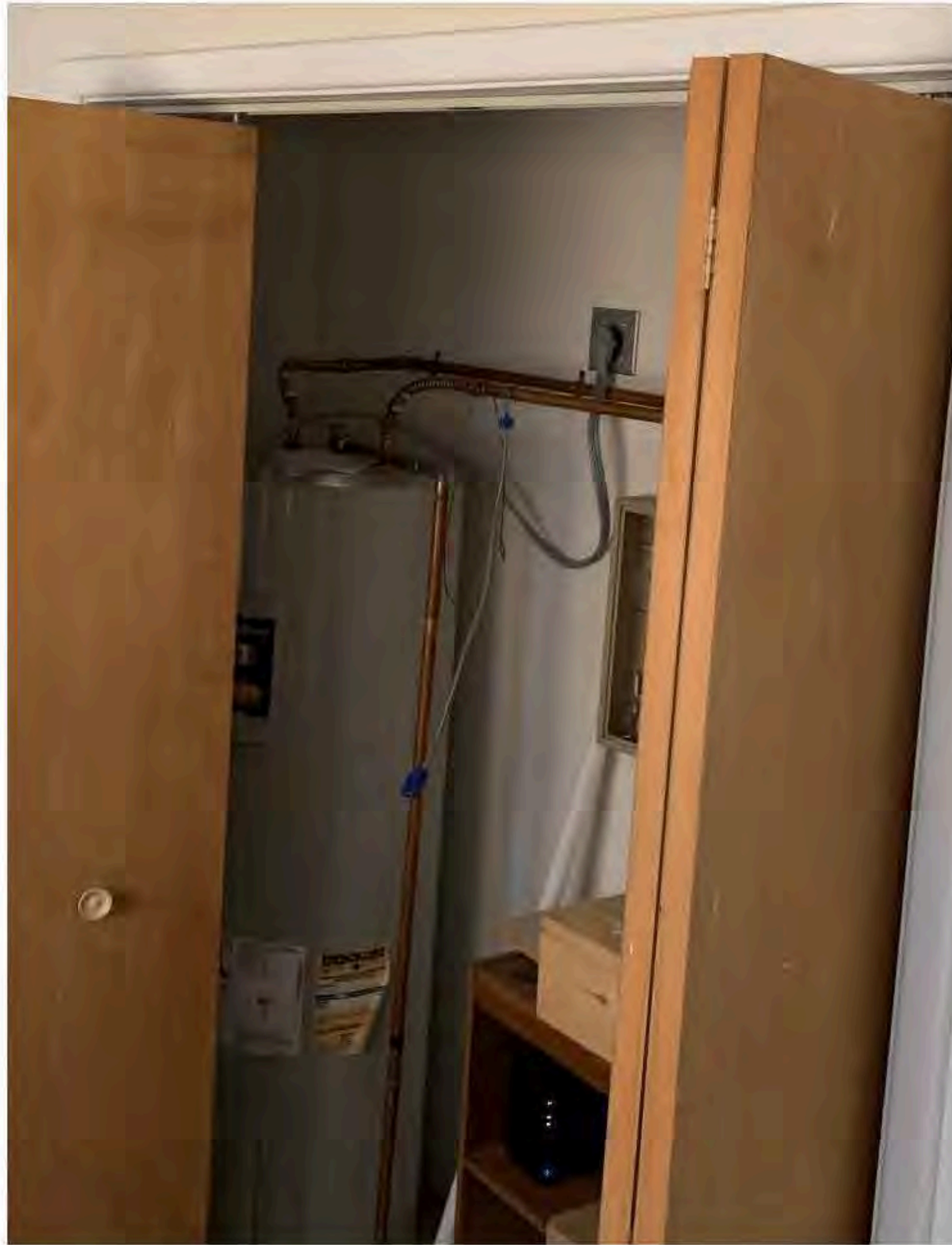
Figure 3.7-4: Upper level closet showing HW heater and copper plumbing
