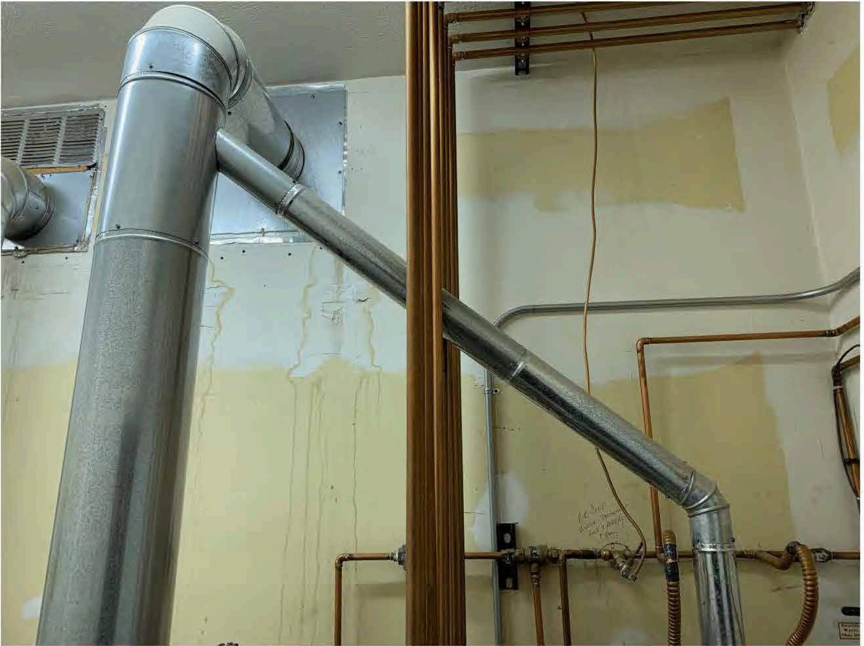
Figure 3.7-2: Hot water boiler and hot water heater flue pipe
