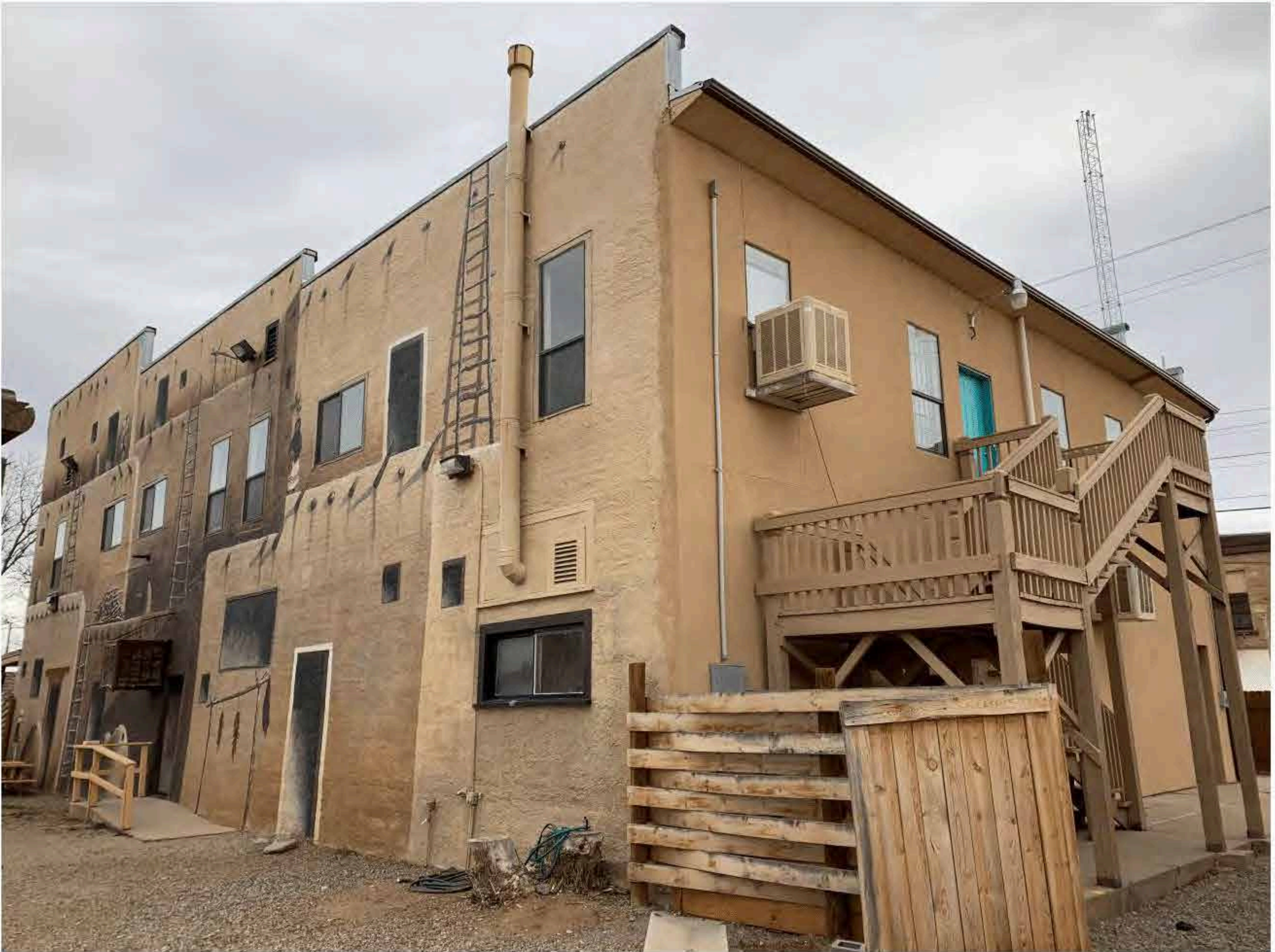
Figure 3.7-3: NW exterior showing 3 evaporative coolers
