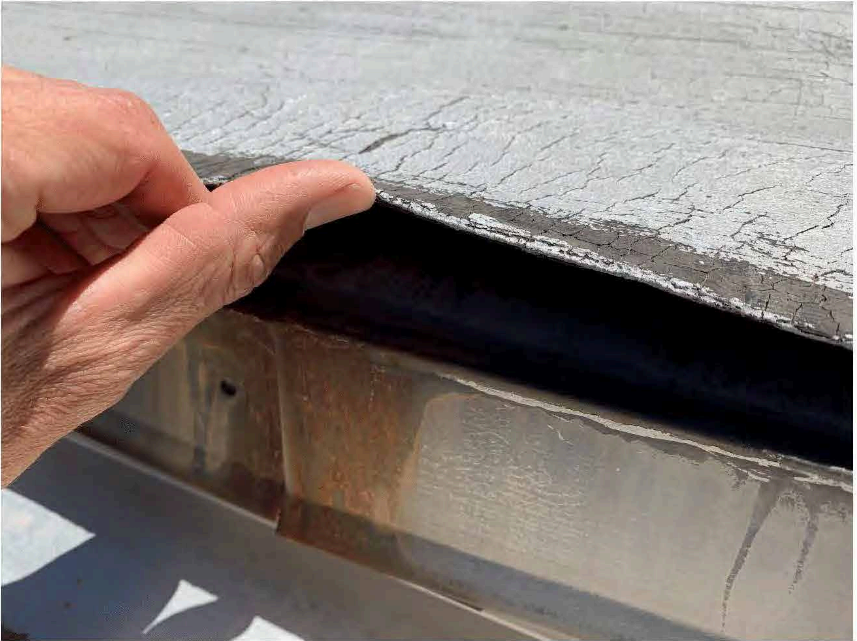
Figure 3.4-4: Drip edge flashing roofing delamination
