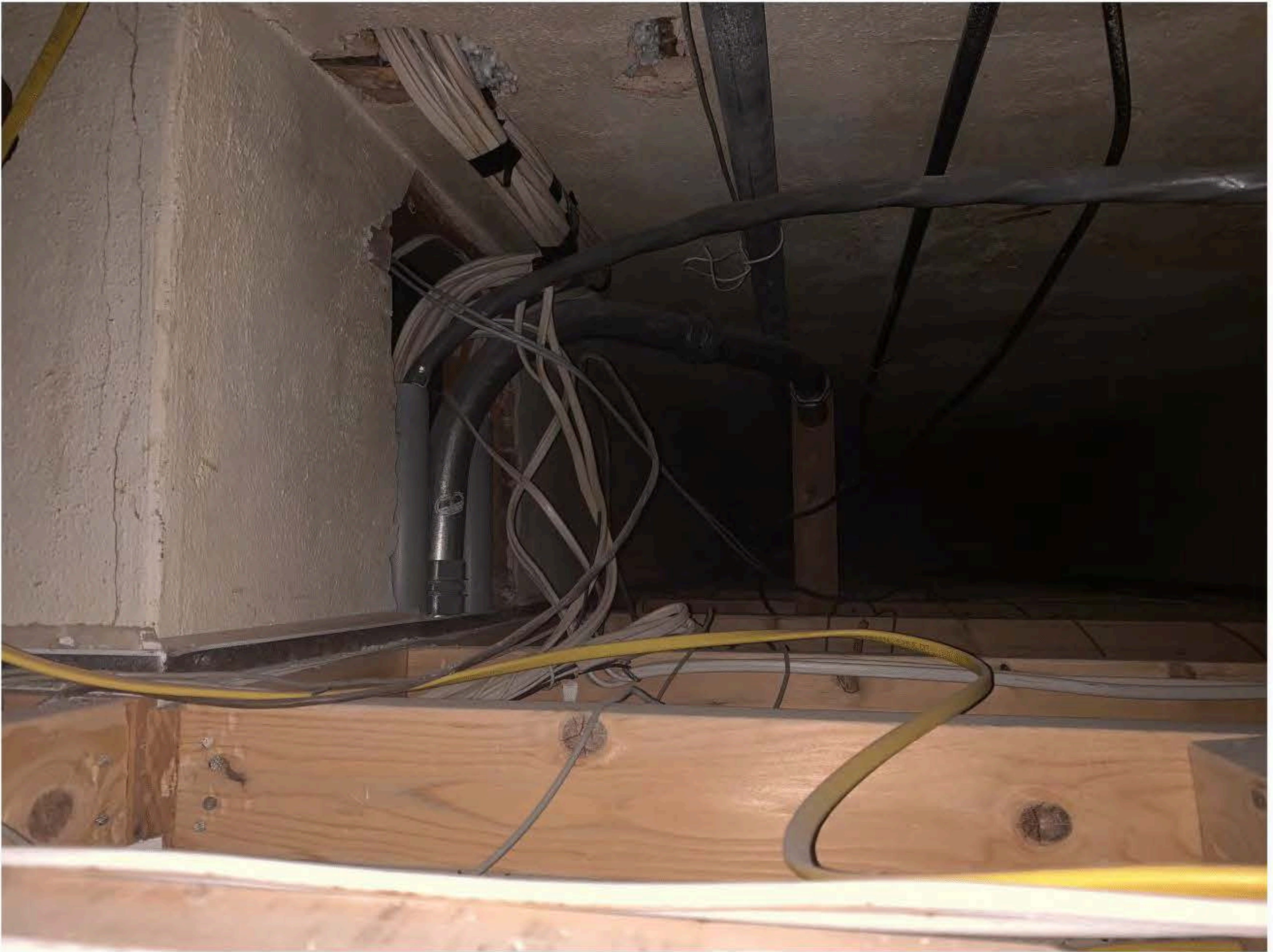
Figure 3.8-4: Upper level wire runs
