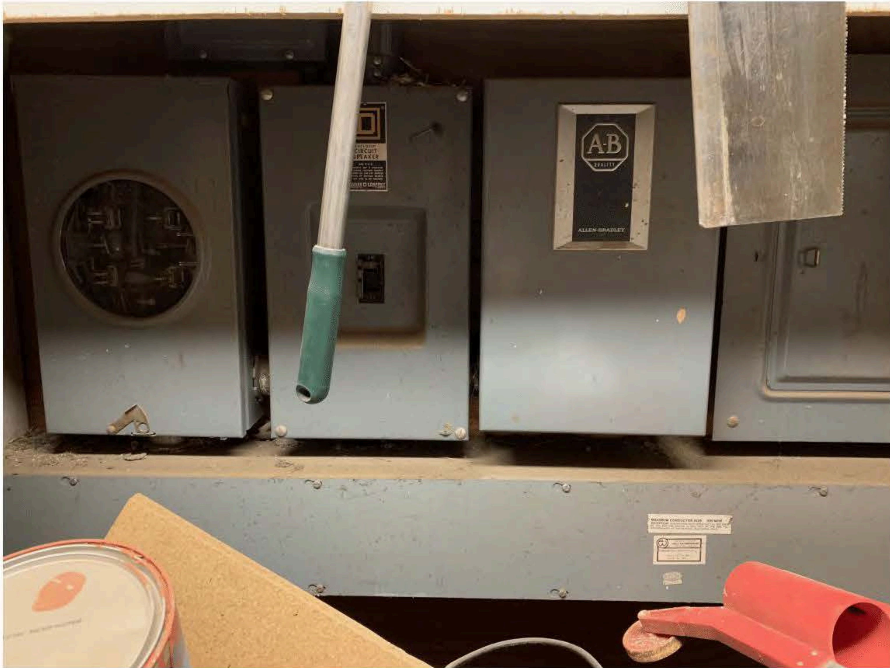
Figure 3.8-2: Main level main breaker panel
