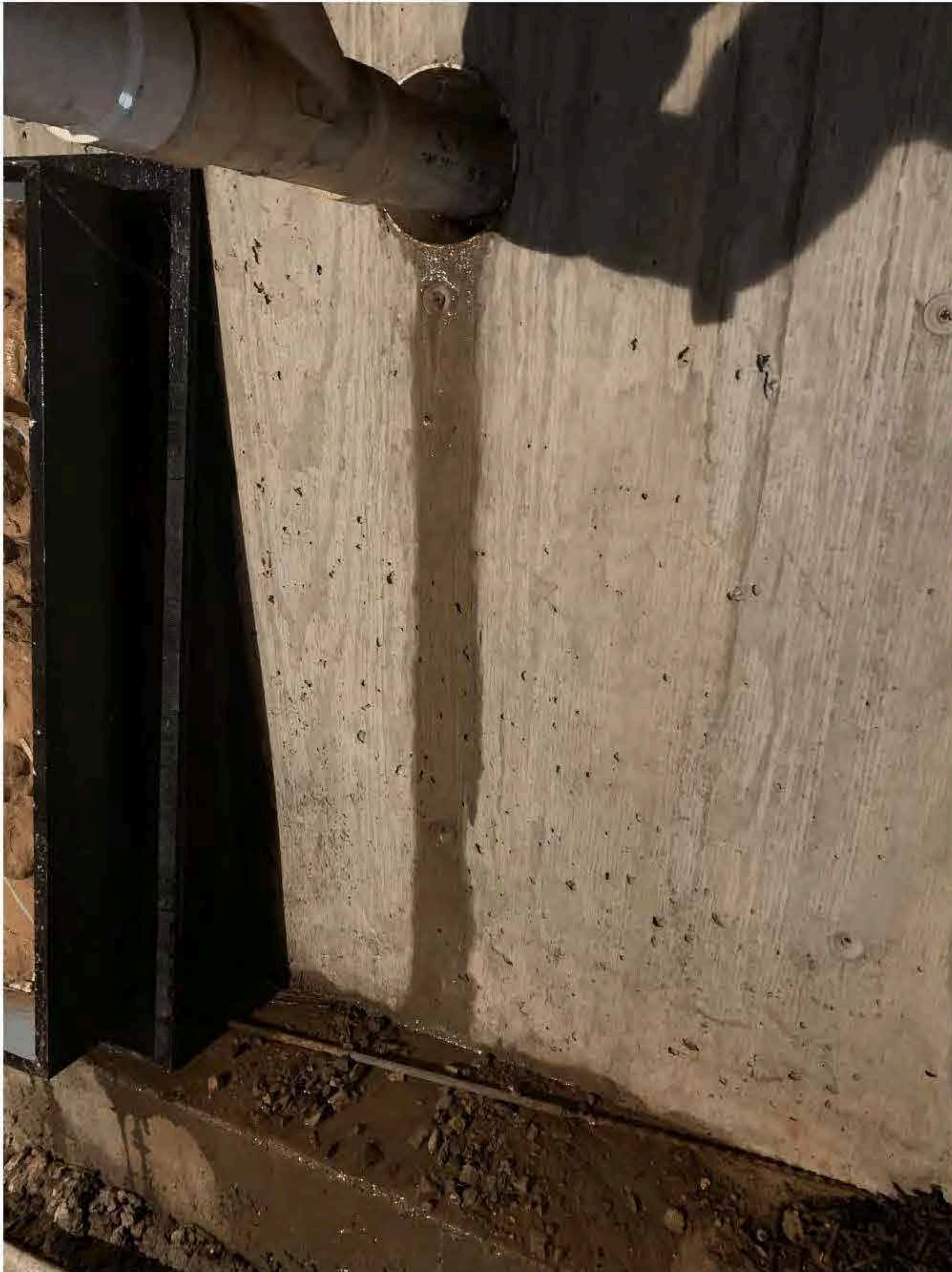
Figure 3.2-3: Leaking sleeve at basement retaining
