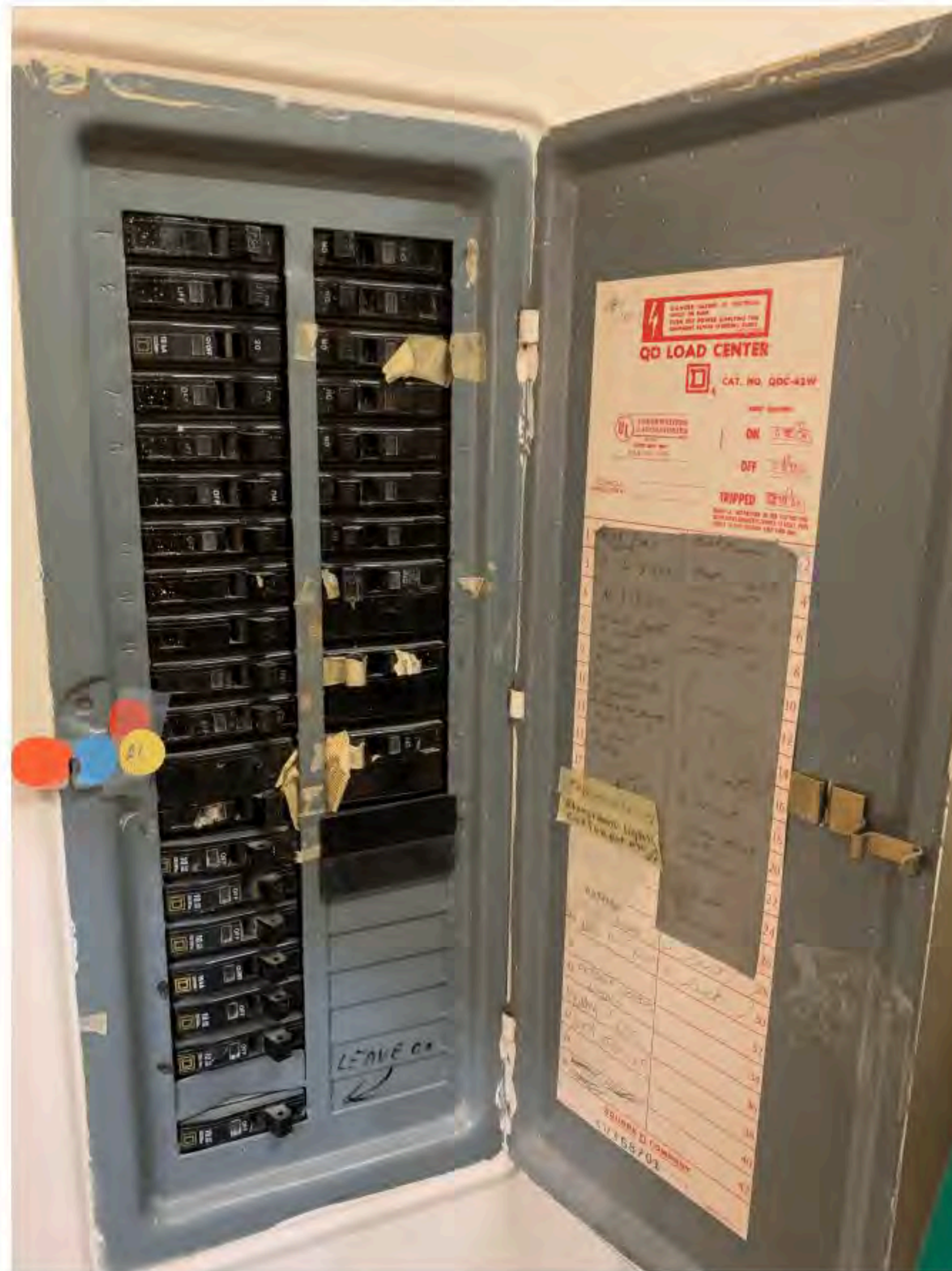
Figure 3.8-1: Main level main breaker panel
