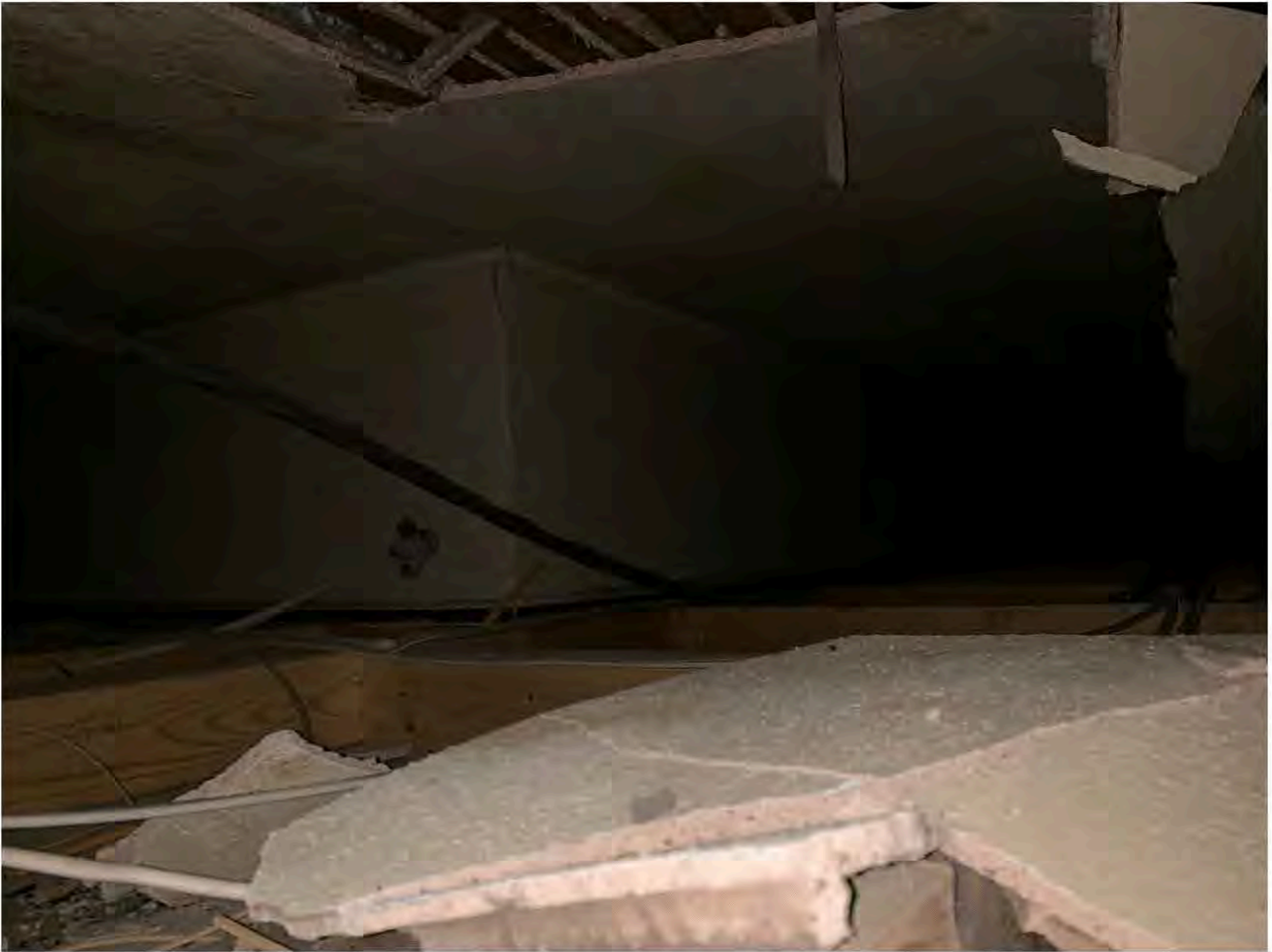
Figure 3.6-7: Dropped GWB ceiling and original lathe and plaster ceiling degradation
